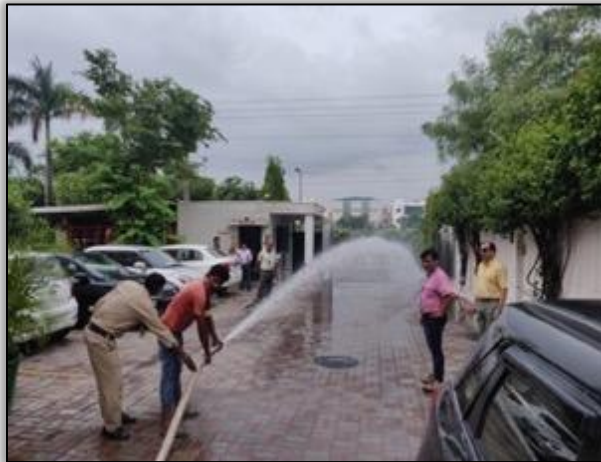
Fire Safety: Fire Hose Reel Pressure Test
