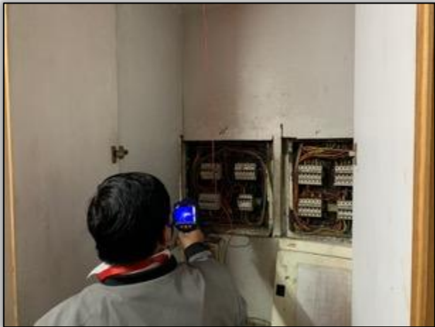
Electrical Safety: Thermo-graphic Test
