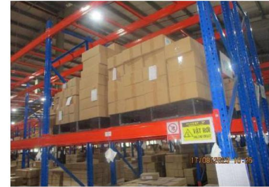
The allowable loading plans were not put on rack and floor of the building
