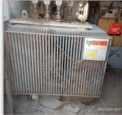
Lint and Dust in Electrical Equipment
