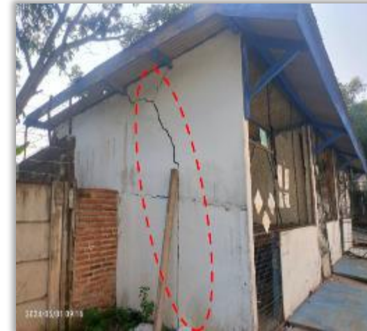
Crack on Non-Structural Member
