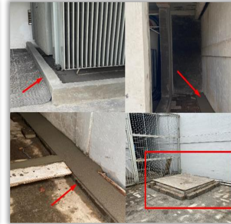
Soak Pit Provided
