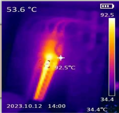
High temperature of 92.5°C observed in electrical panel
