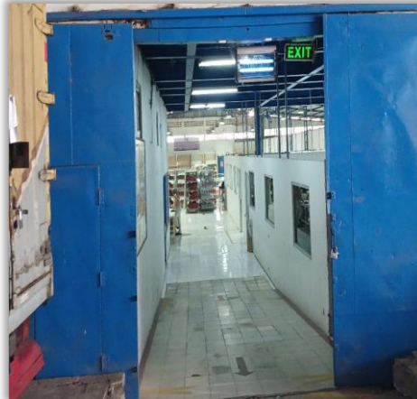
Sliding Doors used as Emergency Exit
