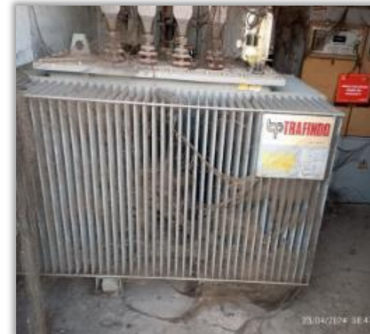
Lint and Dust in Electrical Equipment
