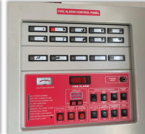
Integrated Alarm System Provided
