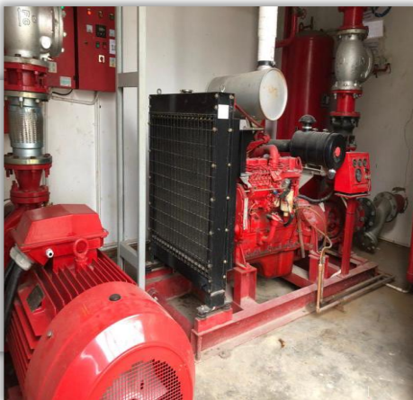
Water Pump Set Provided
