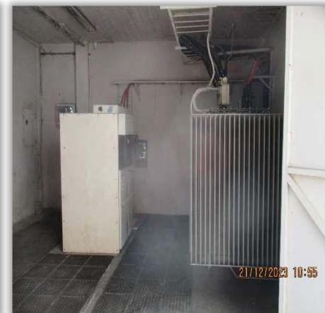
No Oil Soak Pit for Transformer
