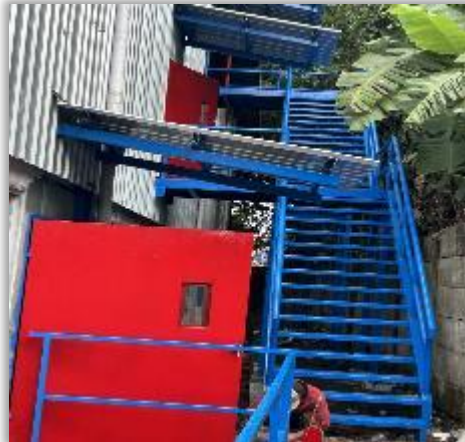
Emergency Exit with FR Door Installed
