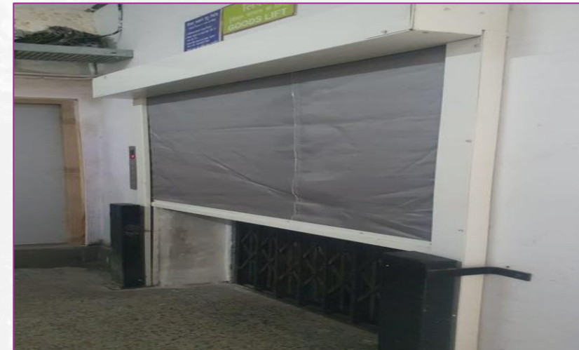
Panel room enclosure by fire door
