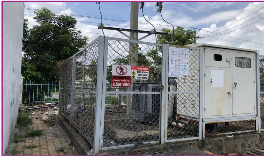
Sign age provided over substation
