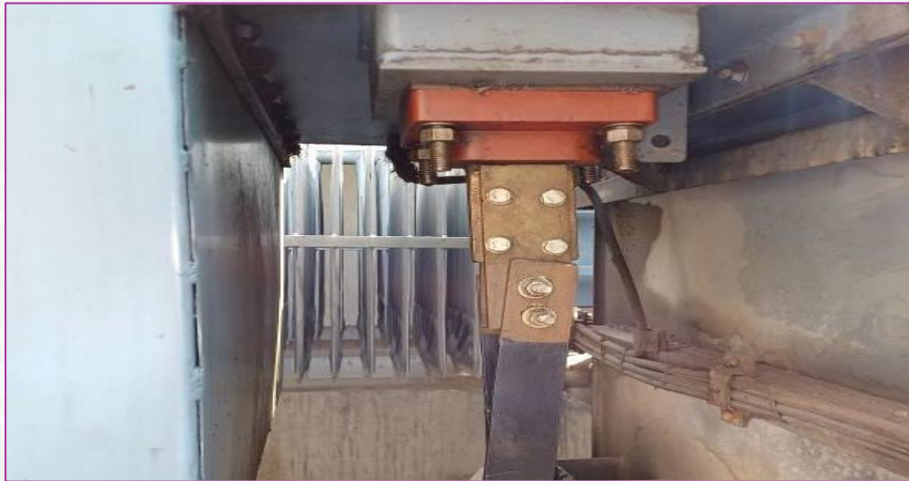
double Earthing provided to transformer
