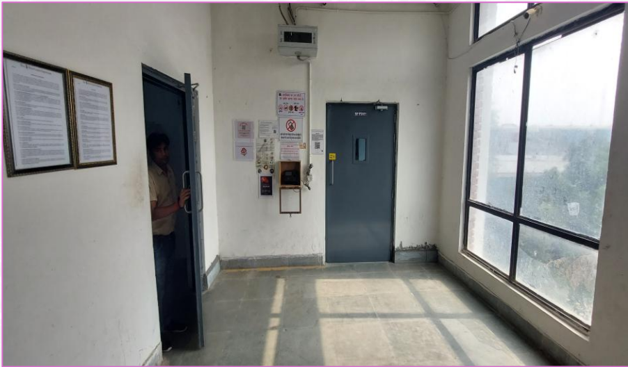
Staircase compartmentation with Fire doors
