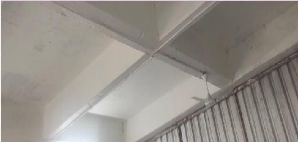
Dampness has been addressed
