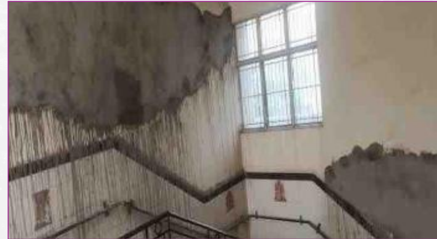
Dampness Repairs work has been done
