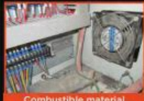
Combustible material inside electrical panel
