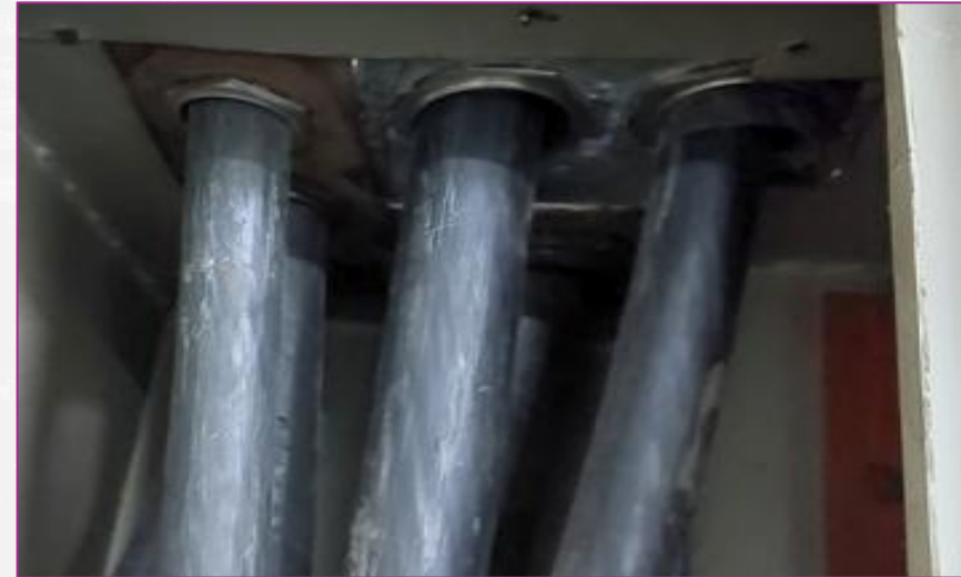
Glands provided over electrical panel
