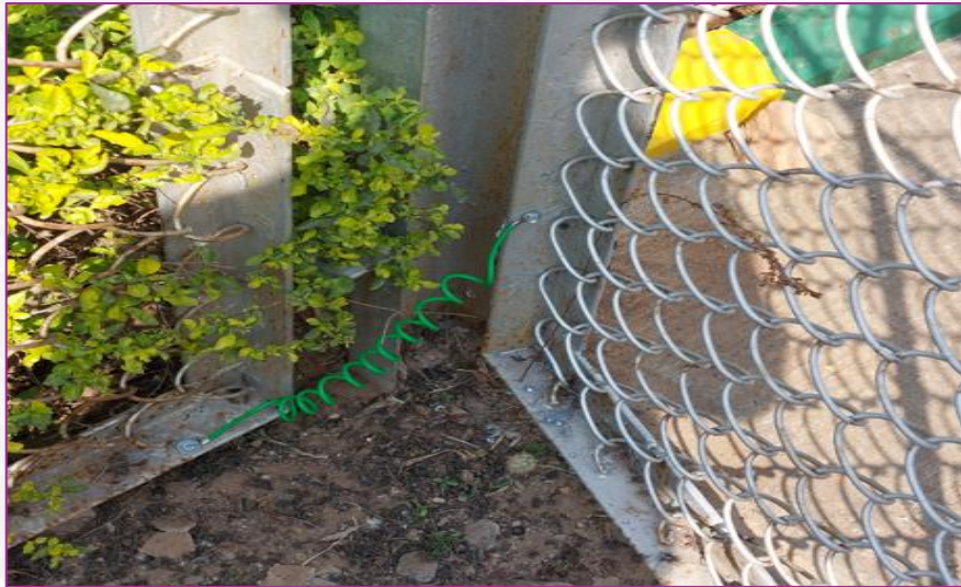
Bonding provided over transformer gate
