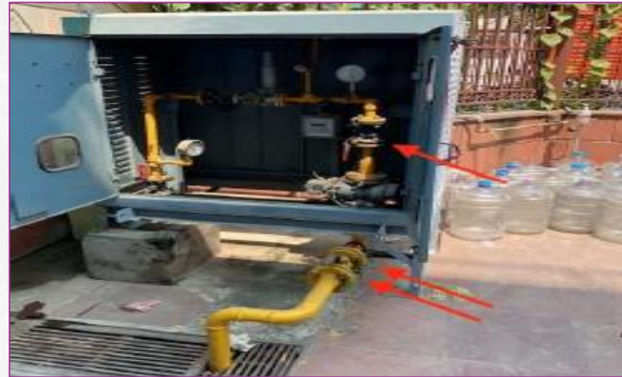
Bonding provided over LPG gas pipeline
