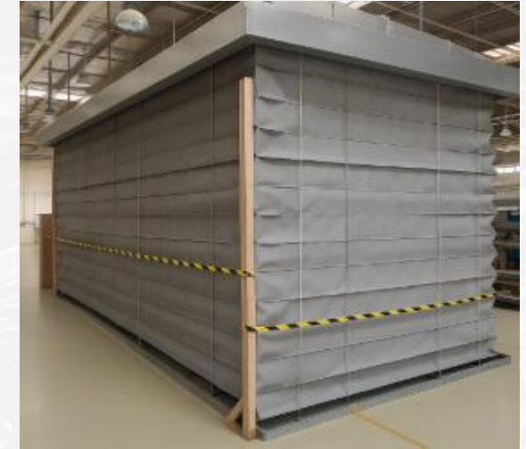
Fire curtain over raw Material Racks
