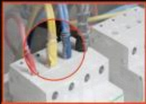
Lint/dirt on electrical panel
