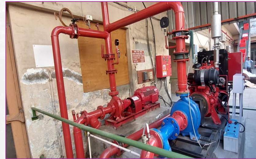
Backup Fire pumps are installed
