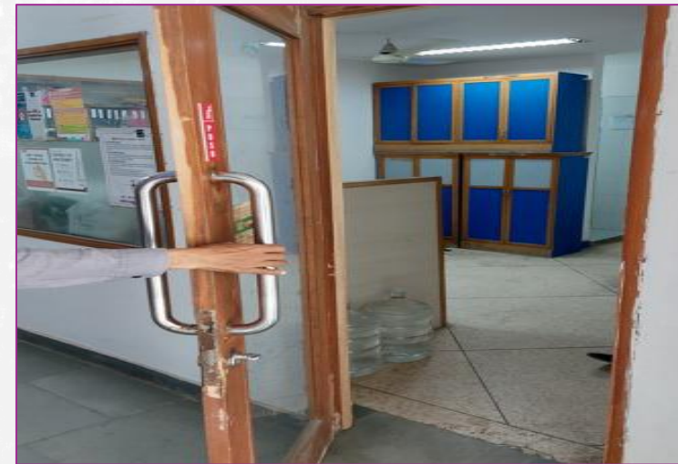
Rotating latch mechanism installed to bypass lock
