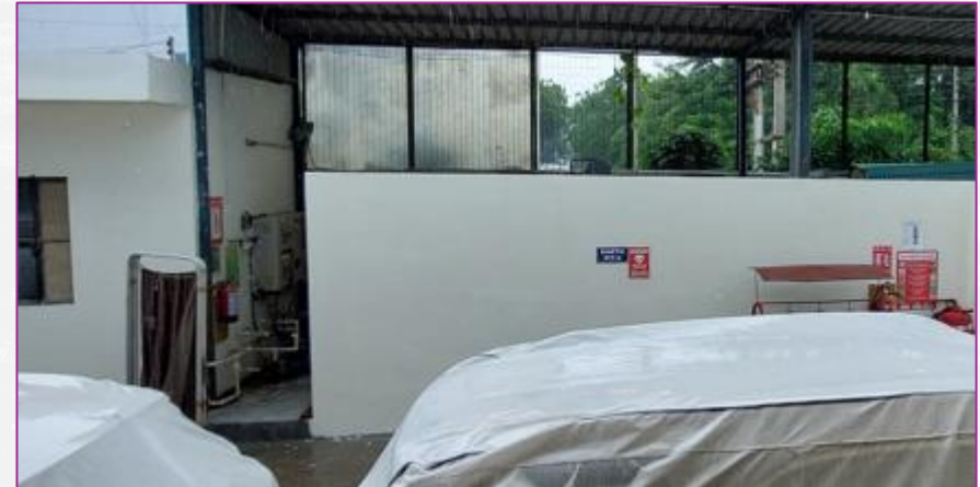
Wall separation provided between transformer & evacuation route
