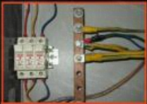
Multi looping of cables
