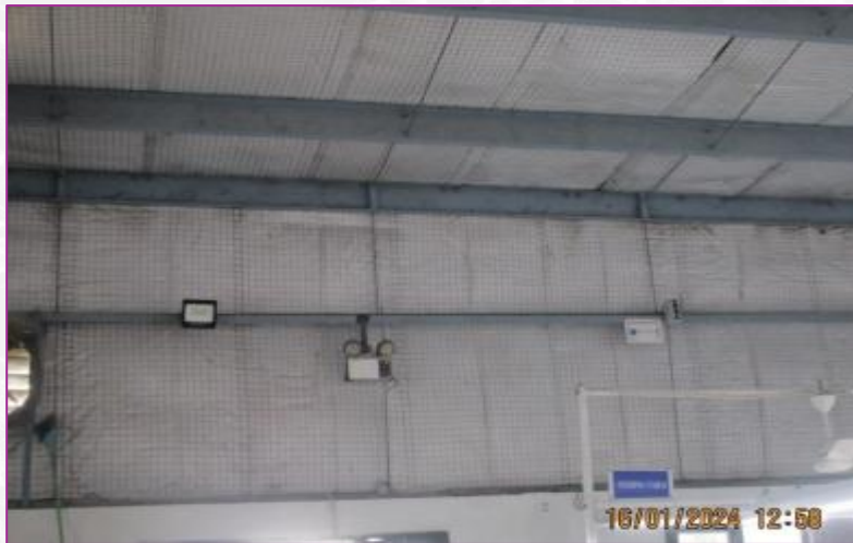
Beam type smoke detector installed for high roof
