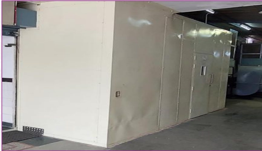
Boiler enclosure by Fire rated material and fire door
