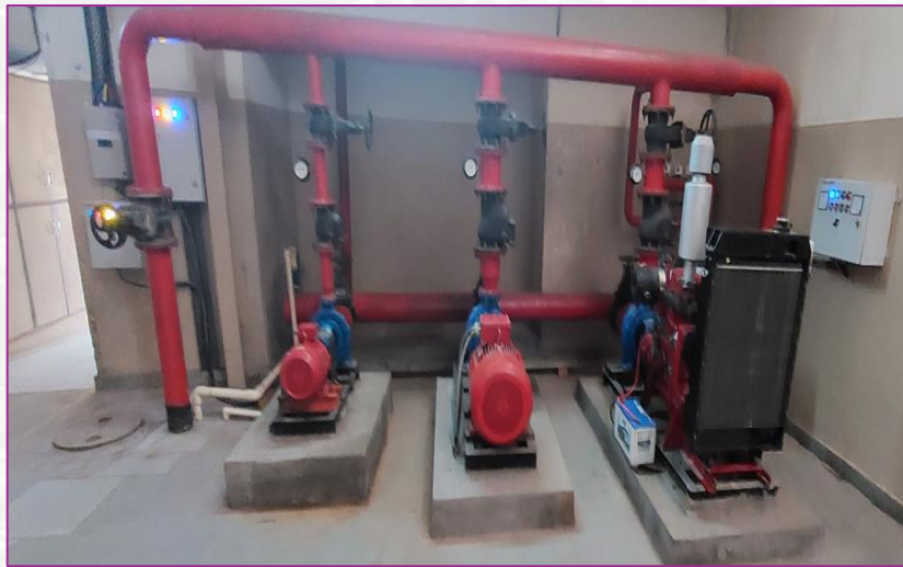
All 3 Fire pumps are installed
