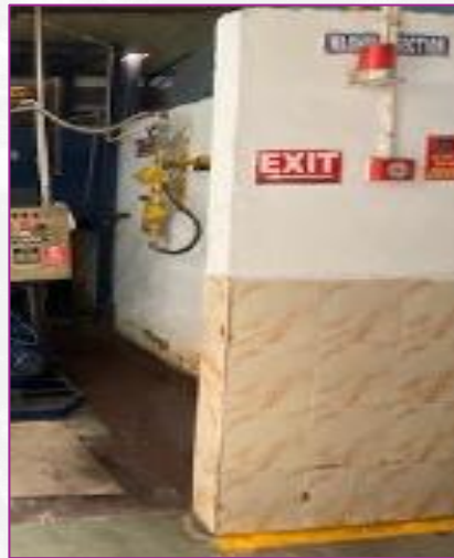
Visual hooters are added in utility area
