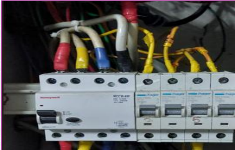
Lugs provided for electrical panel
