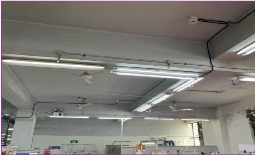
Smoke detector installed
