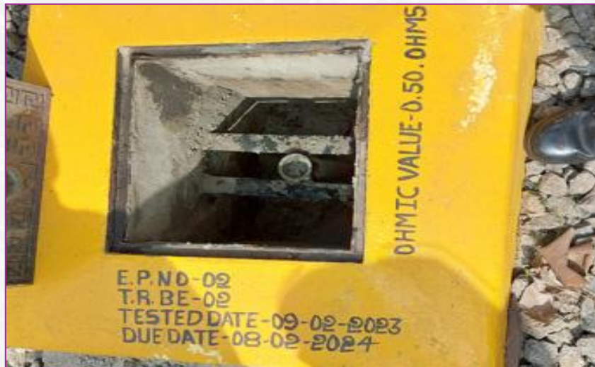
Earth pit maintained and monitored
