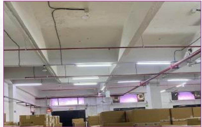
Sprinklers installed in material store
