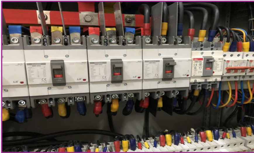
Electrical panel has been cleaned.
