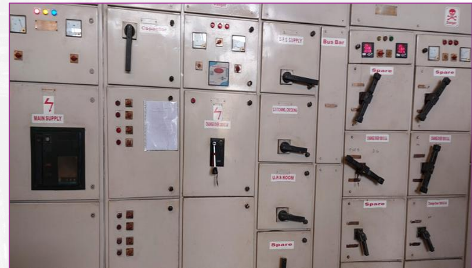
Proper identification provided over panel
