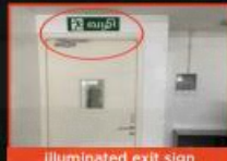
illuminated exit sign not provided over exit
