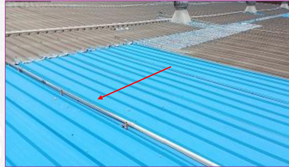
Earthing provided to MS truss
