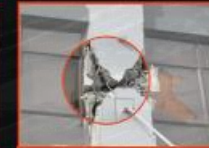
Crack in the pillar
