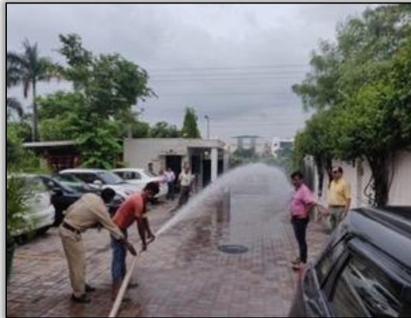
Fire Safety: Fire Hose Reel Pressure Test
