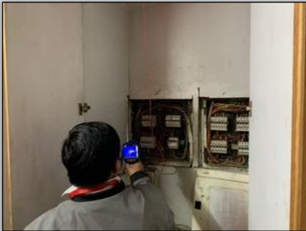
Electrical Safety: Thermo-graphic Test
