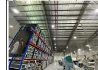
Figure: Drencher system- factory 8, fabric storage
