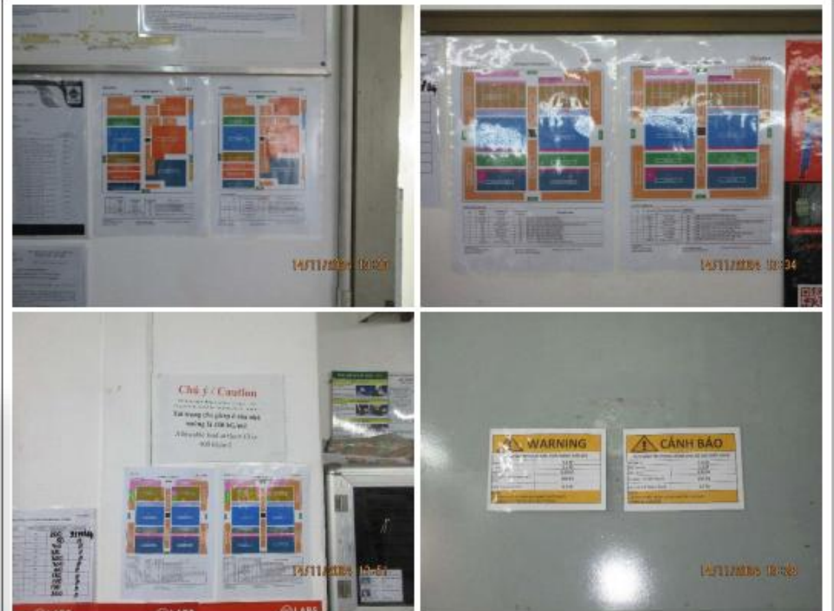
Figure 6: load limit posted at at 1 st floor, 2 nd floor, 3 rd floor and the shelves in the warehouse
