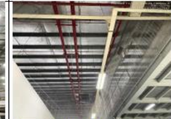
Figure: Drencher system- factory 8, finished goods storage
