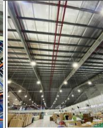
Figure: Drencher system- factory 2
