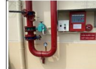
Figure: Drencher system- control panel
