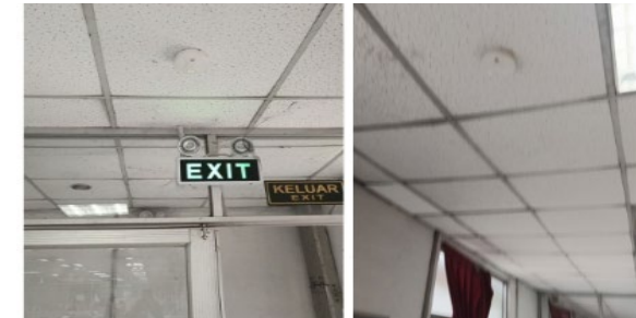
Only Battery Type Fire Detector Installed
