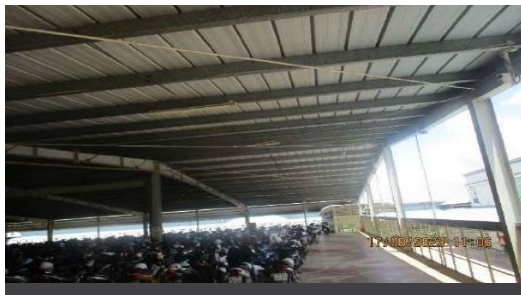
Allowable load limits were not posted on the floors
