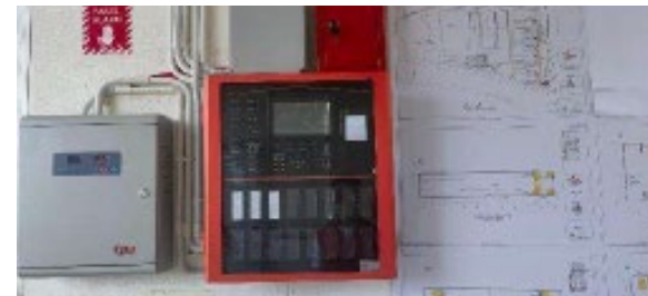
Centralized Fire Detector with Fire Alarm Installed
