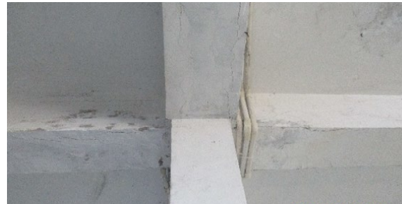
Cracks were observed in beam mezzanine
