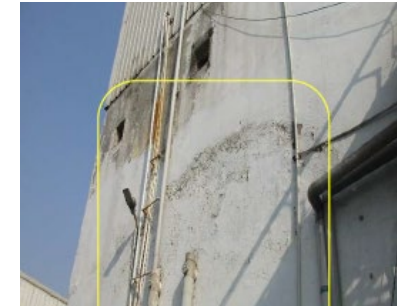
Dampness over building wall
