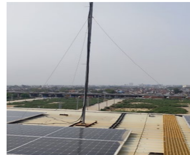
LPS installed over factory building
