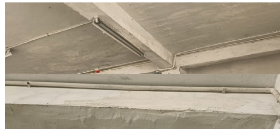
Remediation firm reviewed cracks in the mezzanine beam; the factory then remediate the issue per the firm's recommendations
