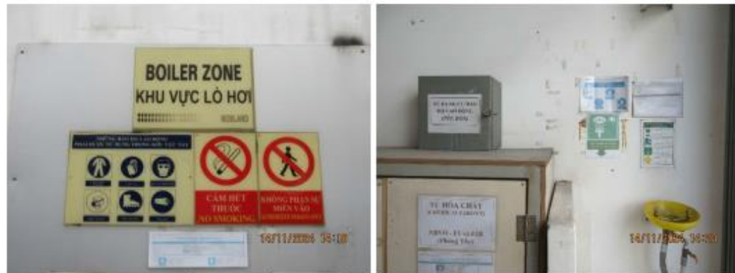
Figure 16.4c: PPE onsite at boiler area and chemical storage
