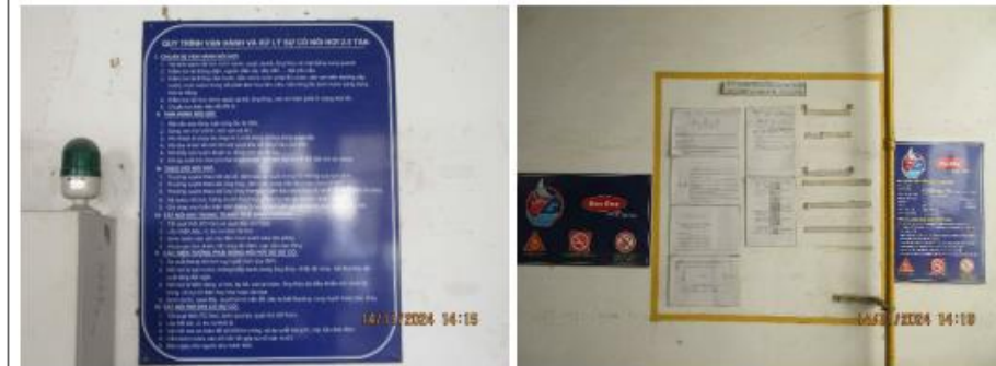
Figure 16.3c: SOPs and checklists posted locally at boiler and LPG station
