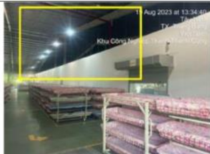
Figure: The warehouse area lacked fire-rated separation from the Production area.
