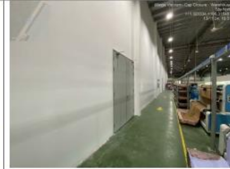
Figure: Self-closing fire rated door on the fire separation of storage and production – Warehouse
