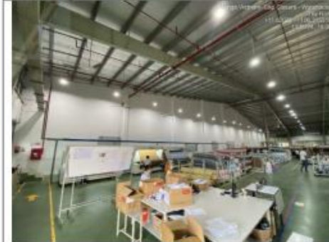
Figure: The fire rated panel 1hours were installed to separate production and storage – production
